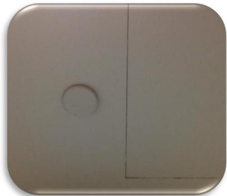
Fire Sprinkler (Concealed)
