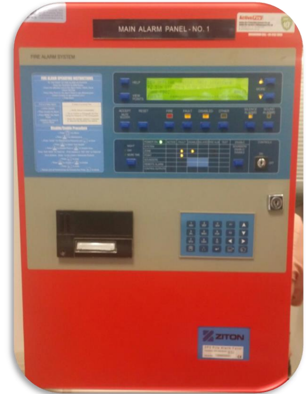
Fire Alarm Panel
