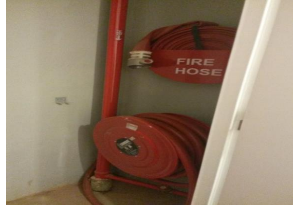
Fire Hose Reel
