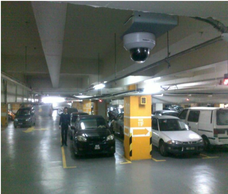
Installation of CCTV camera at strategic location
