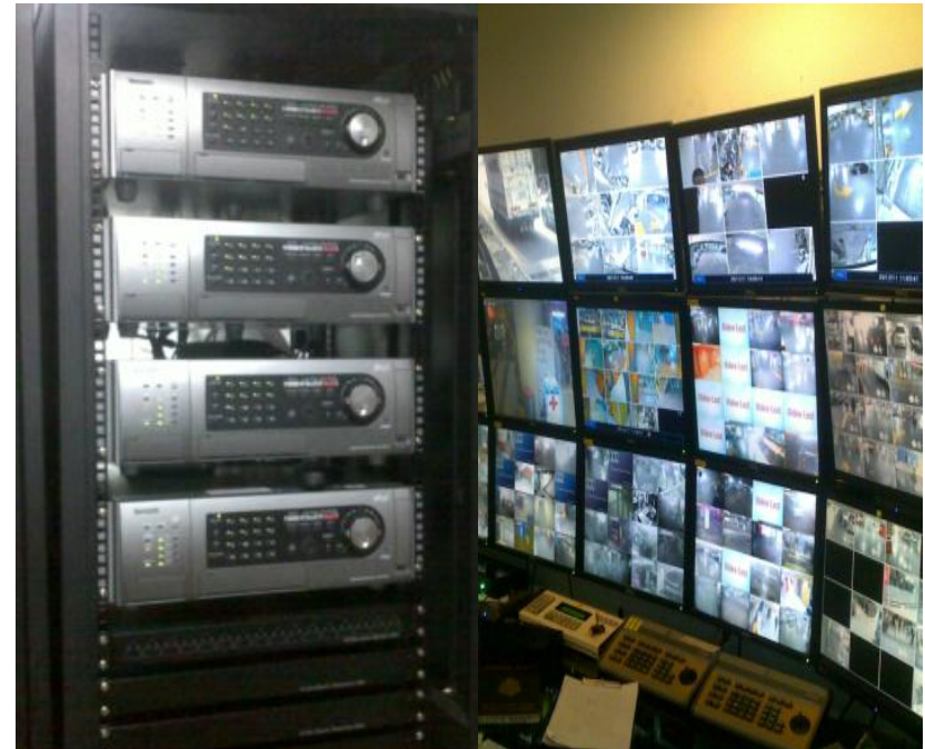
Installation of CCTV monitors and video recorders
