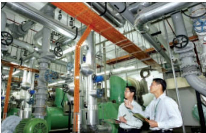
Engineering Services and Energy Management
