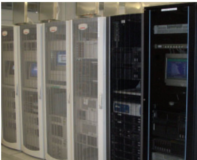
The Data Centre integrates the Group's information flow.
